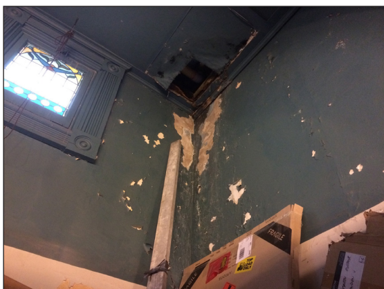
Damaged ceiling in Hammond storage space
